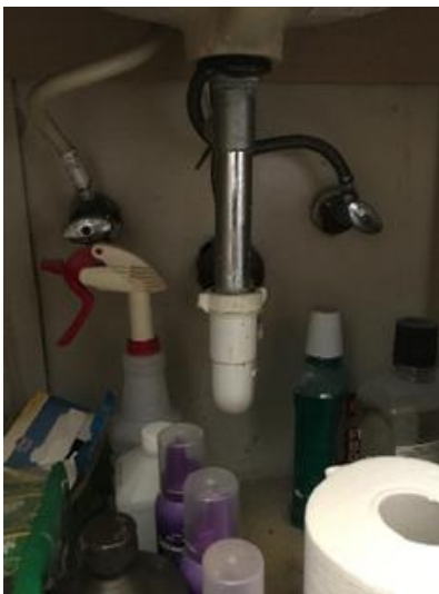
Plumbing/Drain Taken on: 2018-07-30 10:31:39 Taken at: 33.8723454569, -117.90377682 Image
